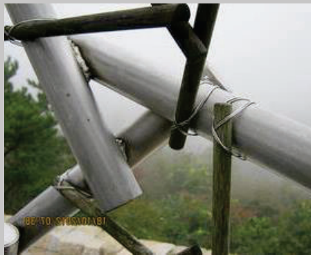
Detail of the welded connection and tied wooden timber battens (photo © Olga Popovic Larsen)
